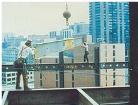
Fig 8 At-risk workers without appropriate safety equipment
